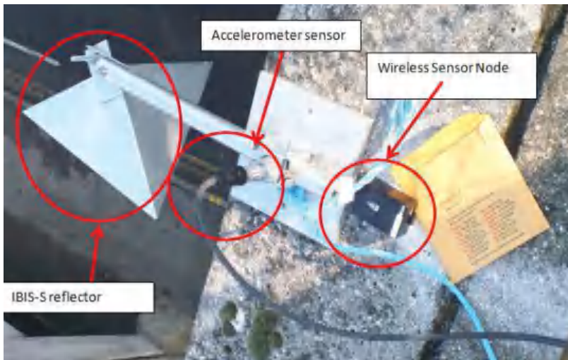
Figure 9. An IBIS-S Reflector, a Wireless Sensor Node and an Accelerometer Sensor
